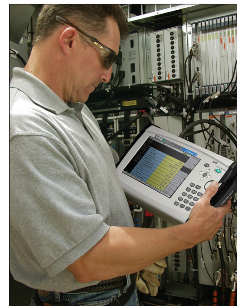
Interference mitigation has often been labor intensive, requiring on-site BTS visits to investigate the problem.
